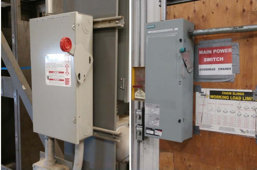
Crane power switches
